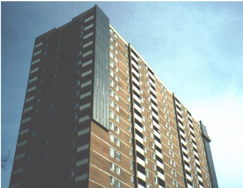
Toronto's twin SolarWall heaters installed at 40 Teesdale Place
