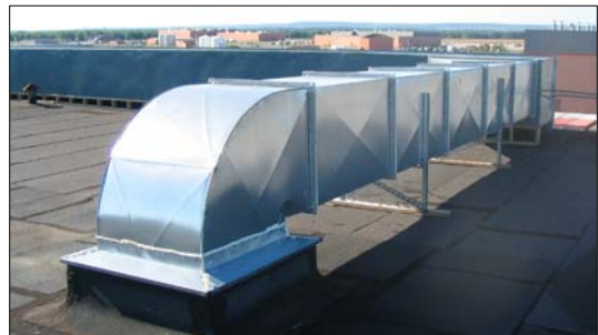
Above, the heat from the SolarWall panels is ducted across the roof to the building's rooftop air intake and HVAC system.
