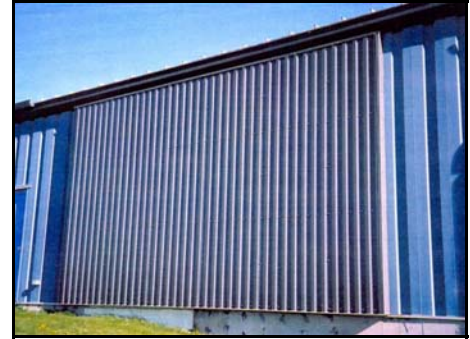
Above: SOLARWALL panels on smaller warehouse wall Left: SOLARWALL panels on main office building and warehouse
